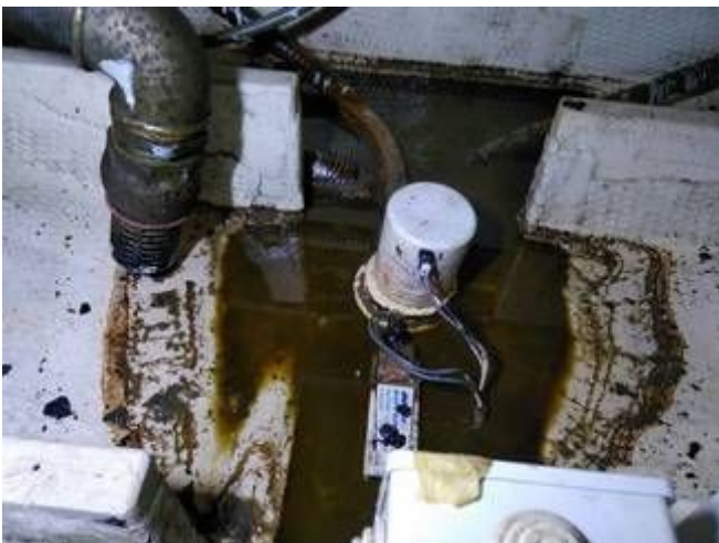
Figura 5: engine room bilge
