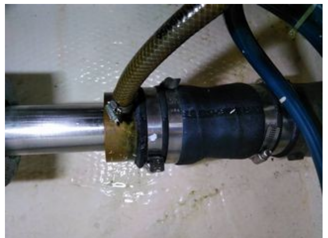
Figura 6: gasoline leak over rubber
